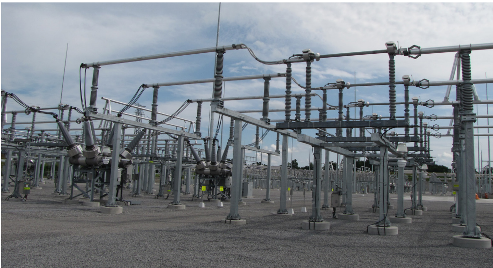
Example of typical switching facility
