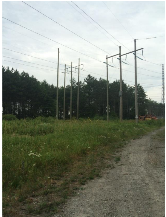
Photo 16: Hydro corridor, disturbance from gravel road, view southeast
