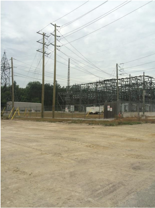
Photo 5: Barrie Transmission Station; view northwest
