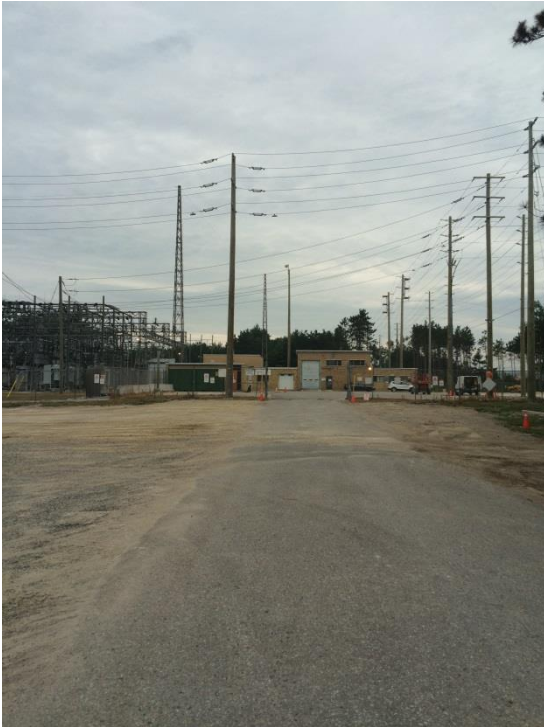
Photo 3: Barrie Transmission Station; view north
