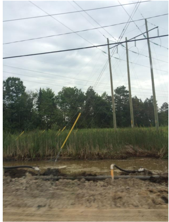
Photo 18: Hydro corridor, ditch flooding associated with ongoing roadwork; view east
