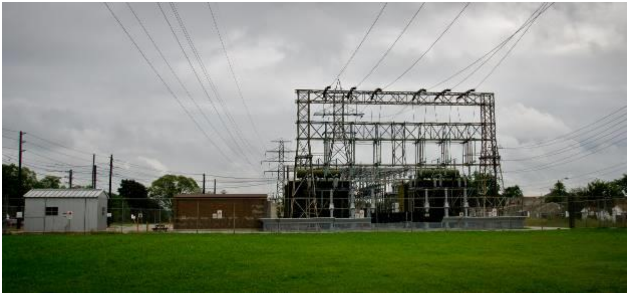
Figure 4: A Typical 115 kV Transformer Station
