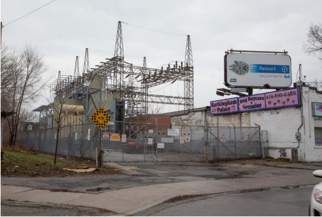
Figure 1-7: Photograph of Main TS
