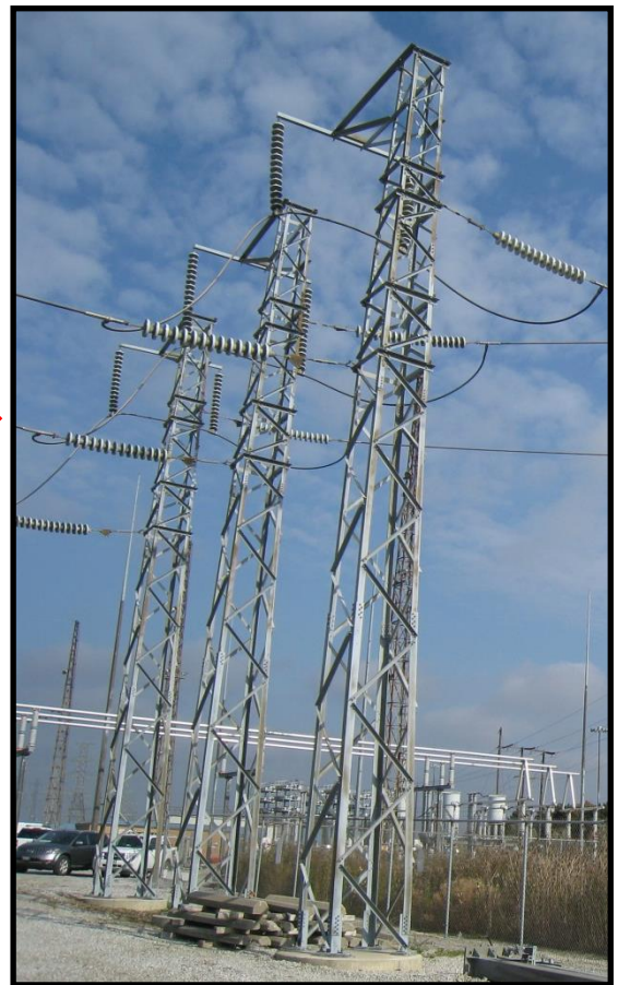
New Tapping Structures
