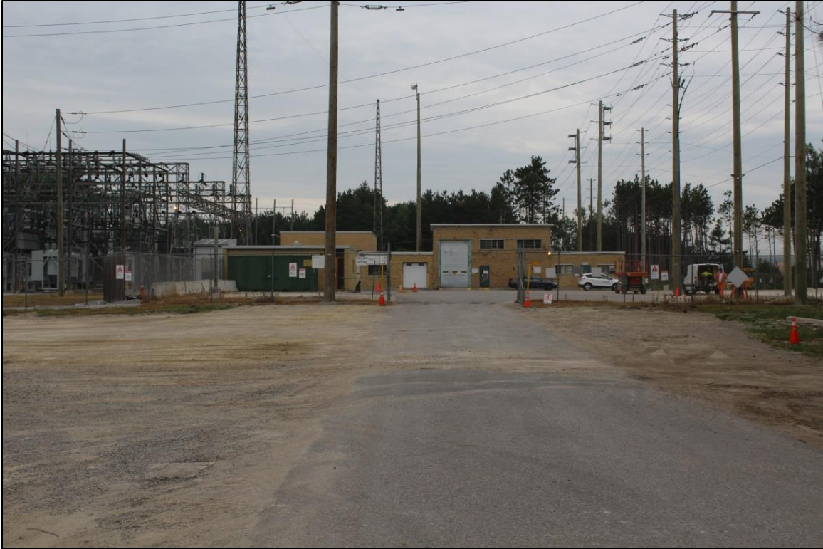
Figure 3: View to north of Hydro One Transmission Station
