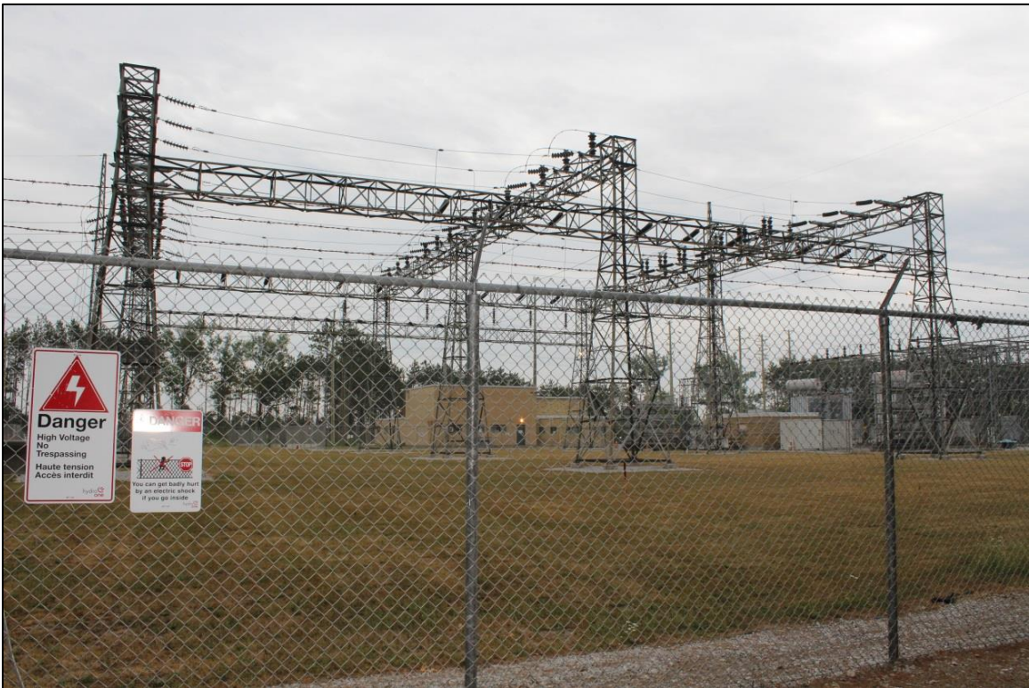
Figure 4: View to south east of Hydro One Transmission Station
