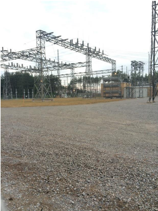
Photo 11: Barrie Transmission Station, disturbed from construction; view northeast
