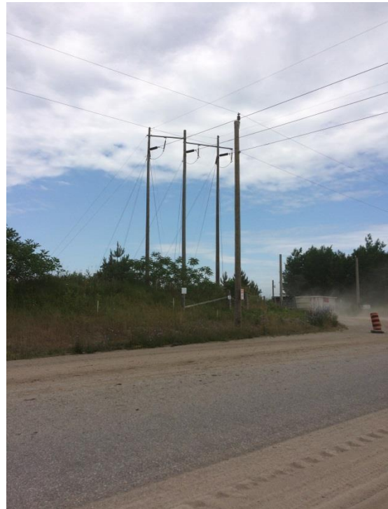
Photo 28: Hydro corridor through active quarry. No permission to access, condition of property unknown; view northwest
