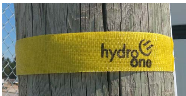
Figure C: Yellow Tag for Defective/Deteriorated Hydro One Poles
