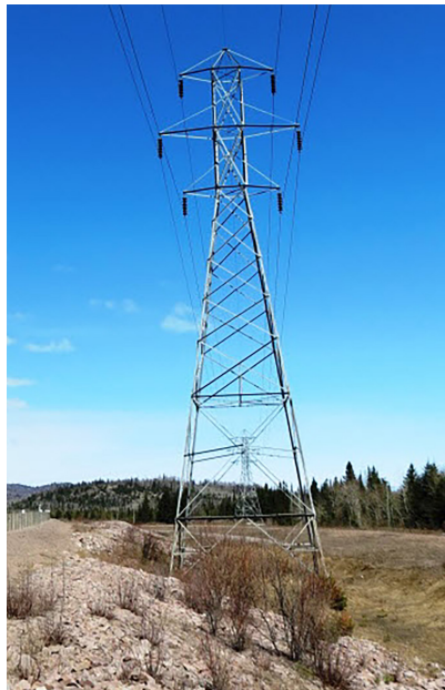
115 kV Steel Structure (A7L/R1LB Transmission Line)
