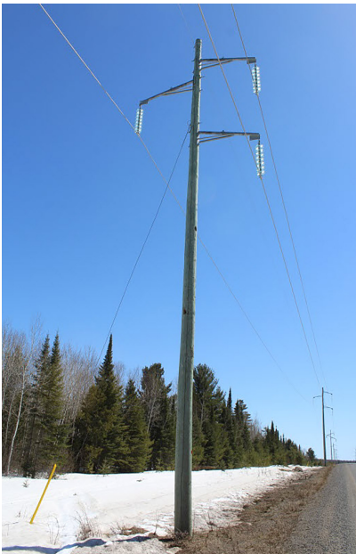
115 kV Wood Pole Structure (A6P Transmission Line)
