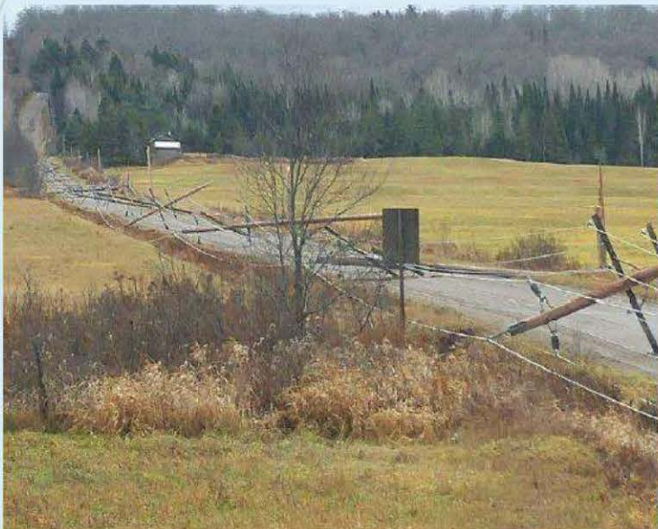
(Above) Over 40 broken poles along the route to Burks Falls DS near Huntsville were toppled over by the wind storm.
