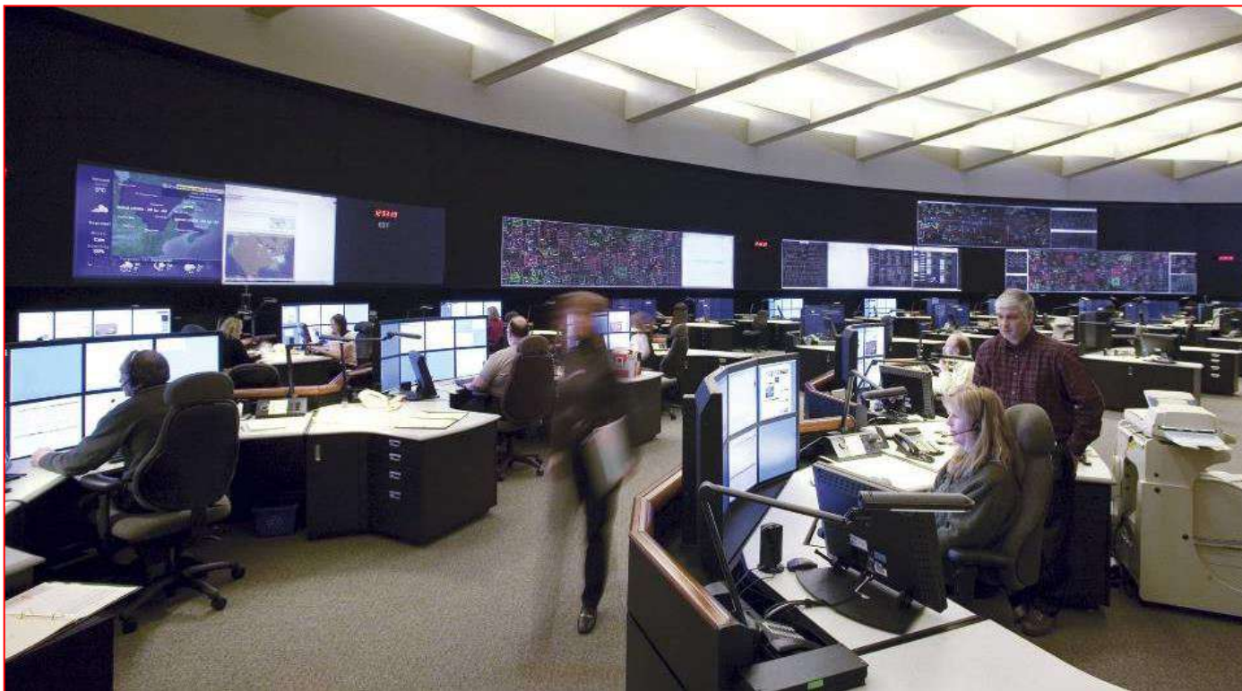
Operating the Transmission and Distribution systems of Hydro One
