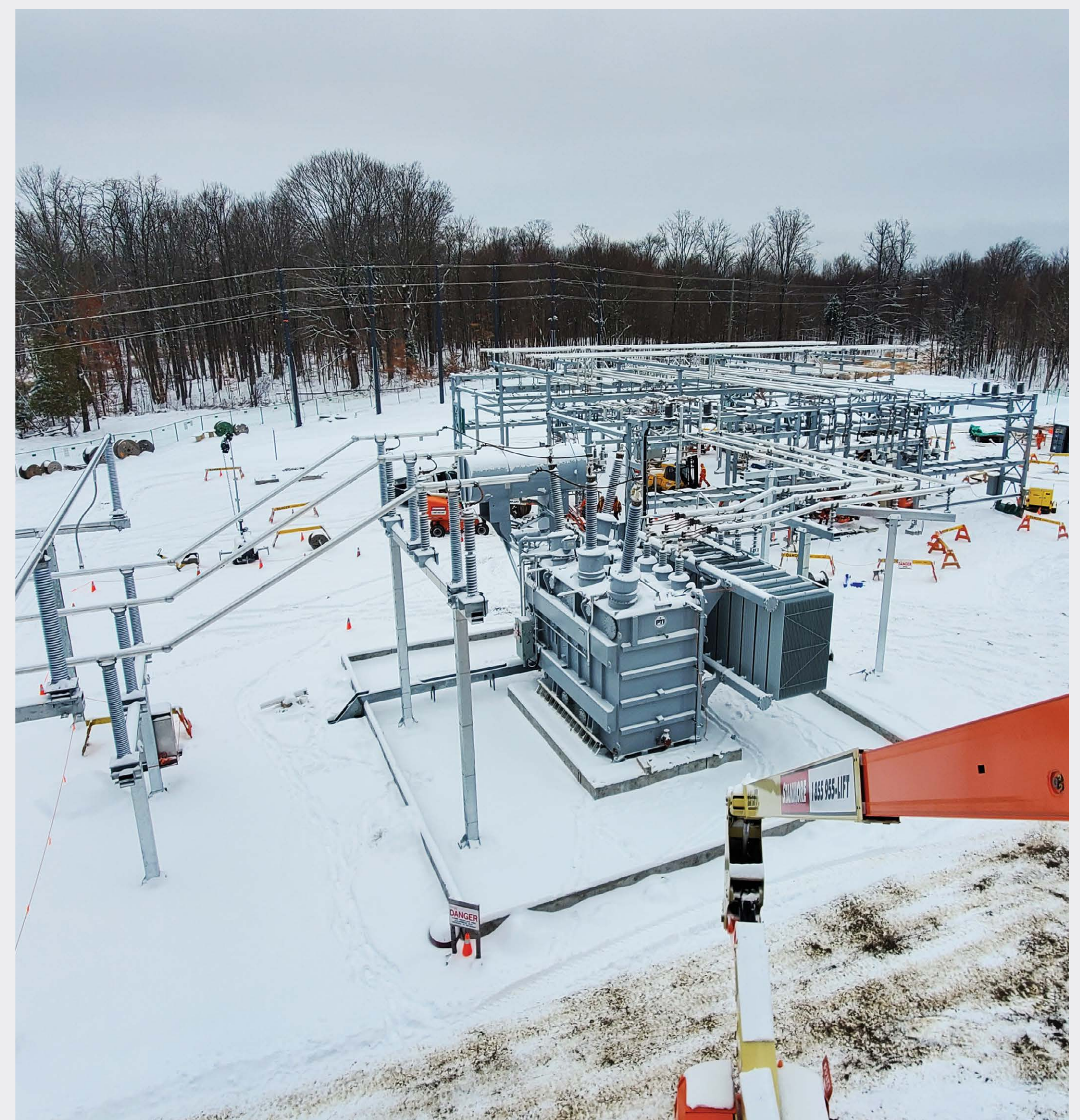
Example of Transformer Station
