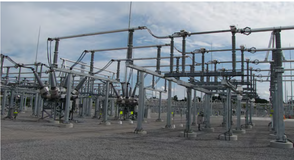
Example of typical switching facility
