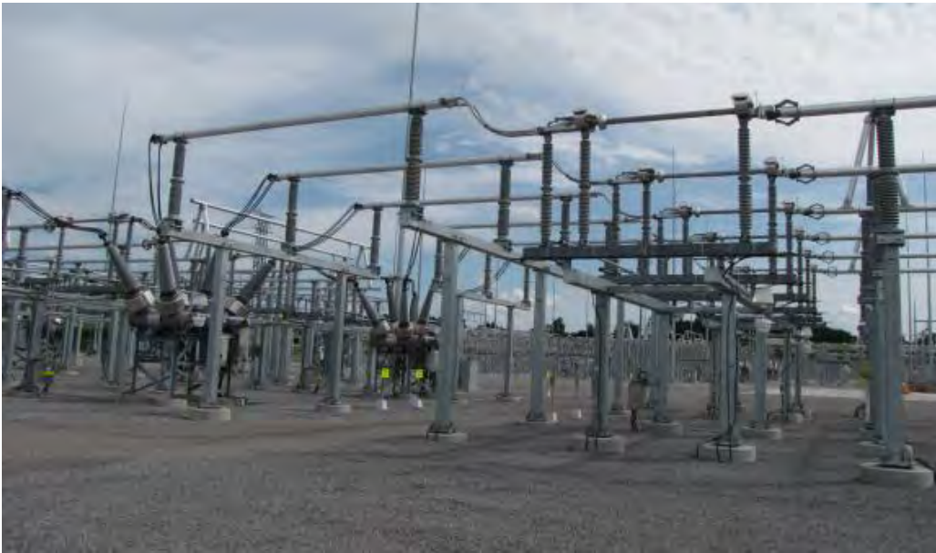
Figure 6-1: Example of Typical Switching Station
