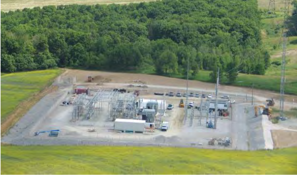
Figure 6-2: Example of Typical Transformer Station
