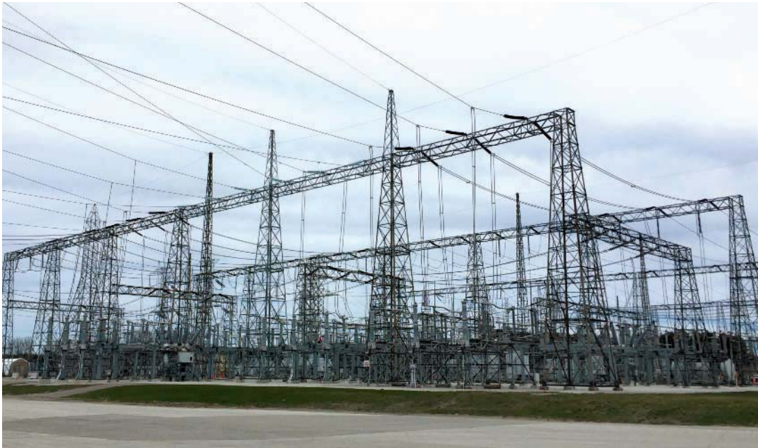
Current view inside Essa TS
