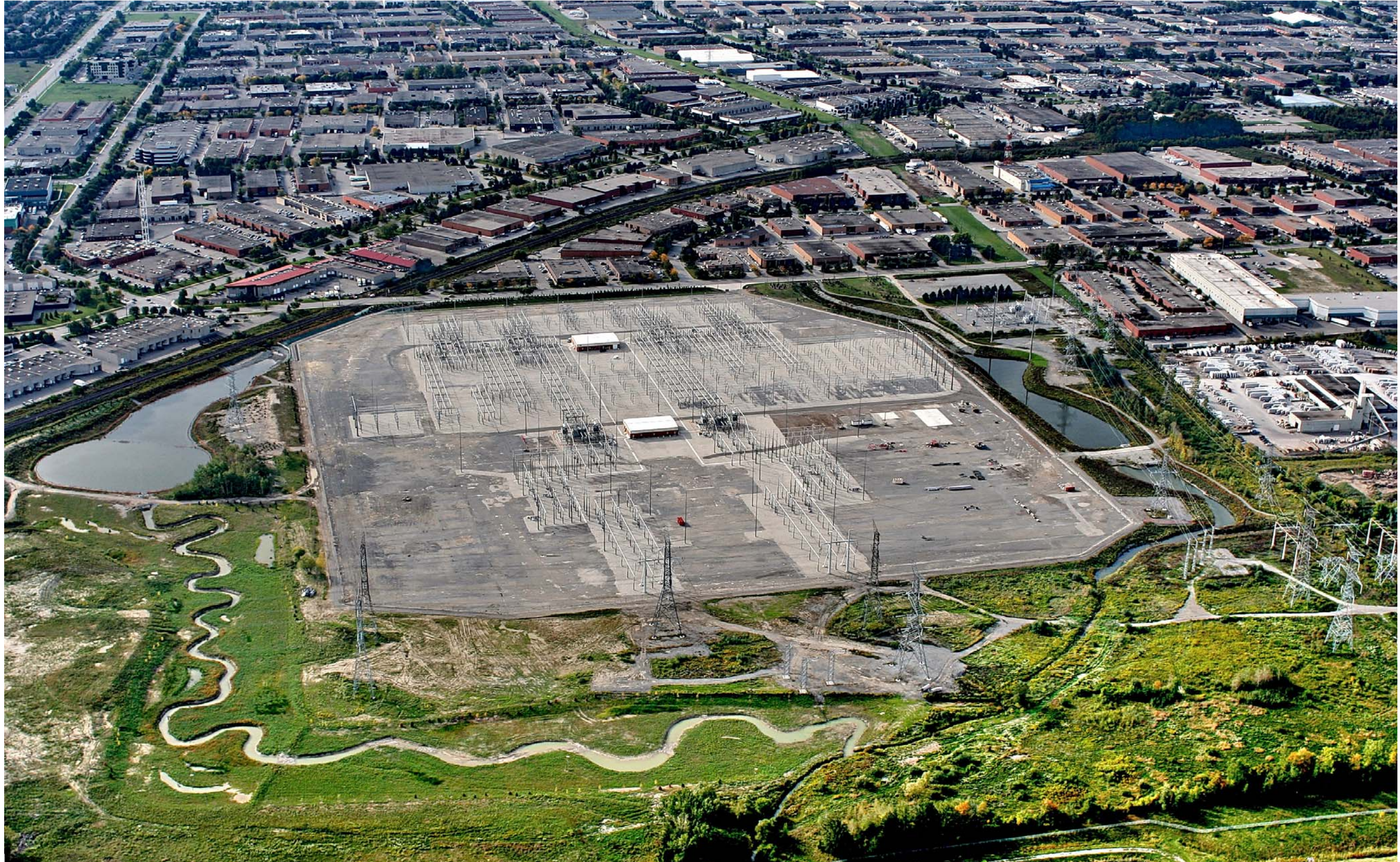
Figure 1-4: Parkway Transformer Station
