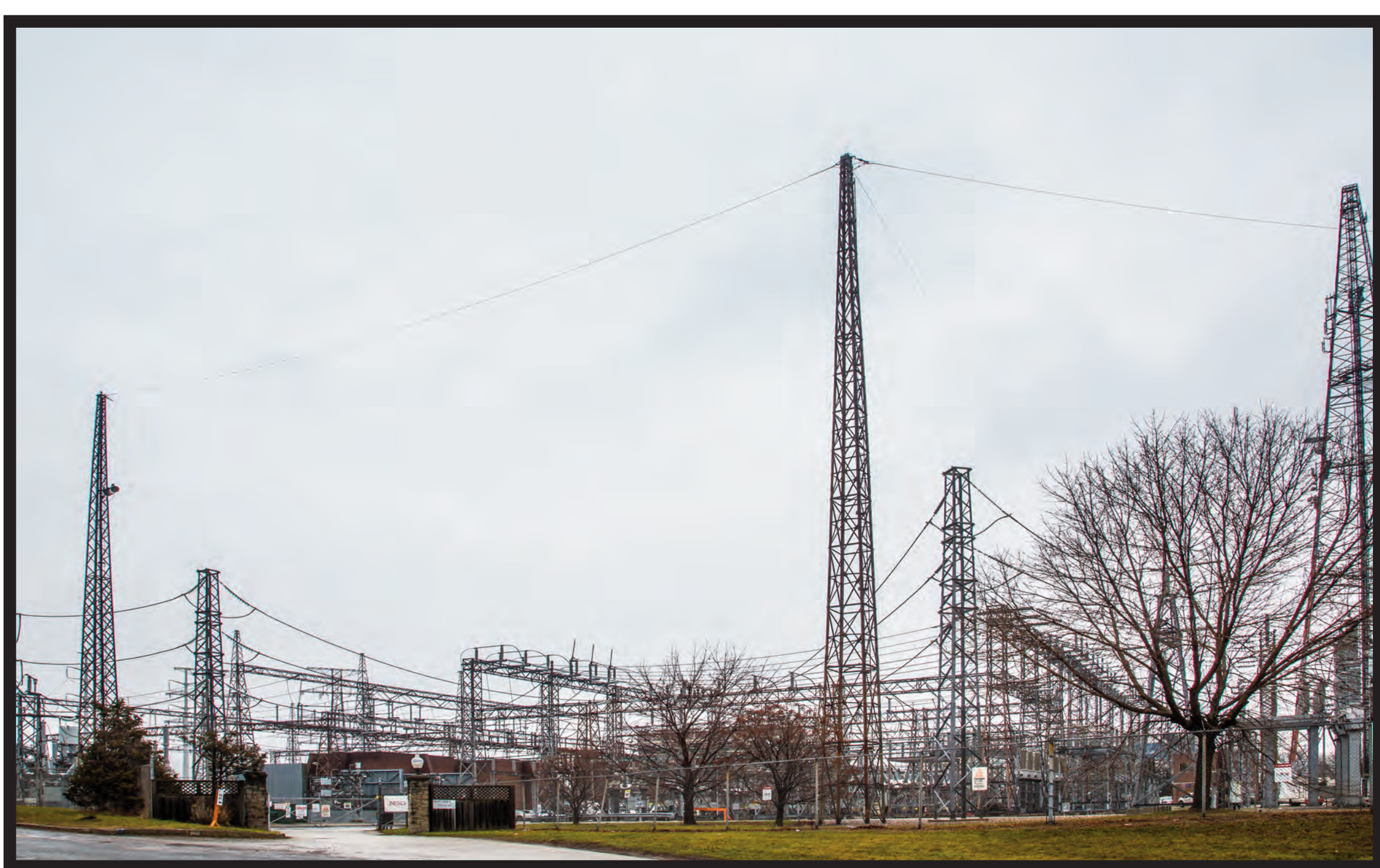
Leaside Transformer Station
