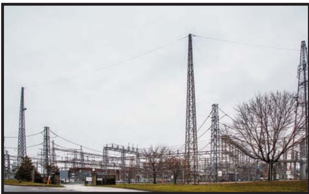
Leaside Transformer Station
