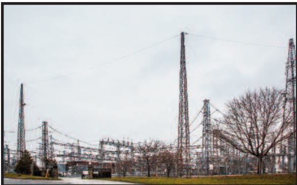
Leaside Transformer Station
