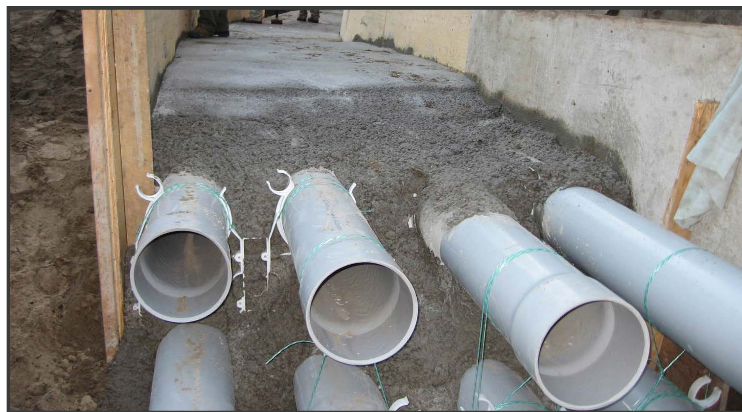
Example of cable ducts
