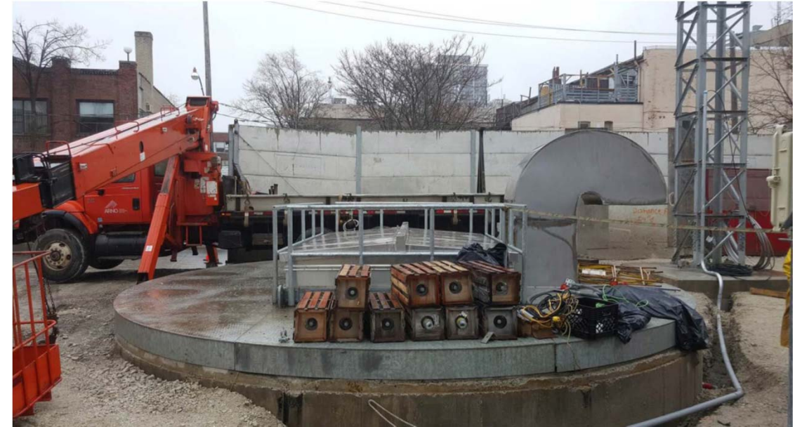
Example of access shaft
