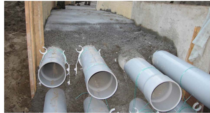
Example of cable ducts
