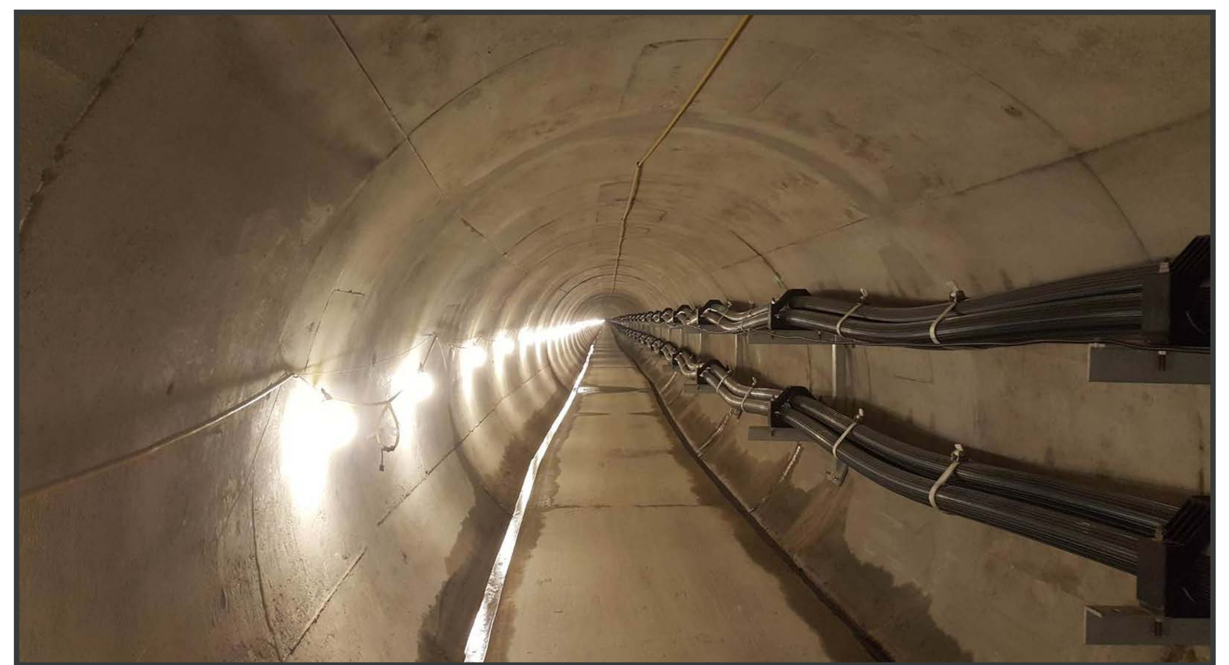
Example of underground tunnel with cables
