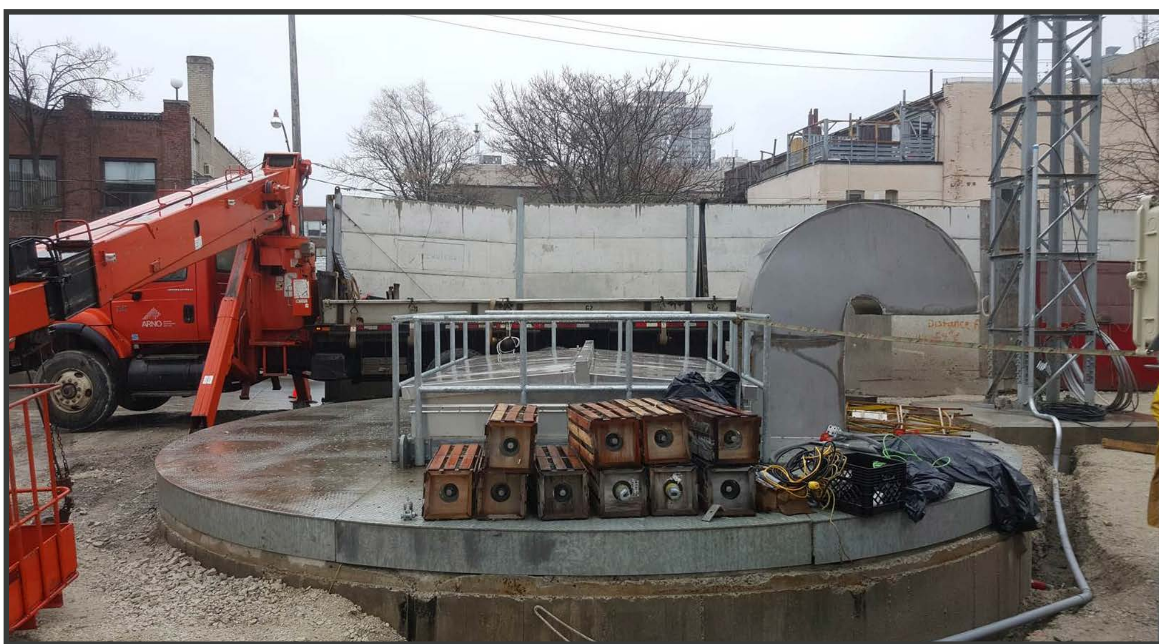
Example of access shaft
