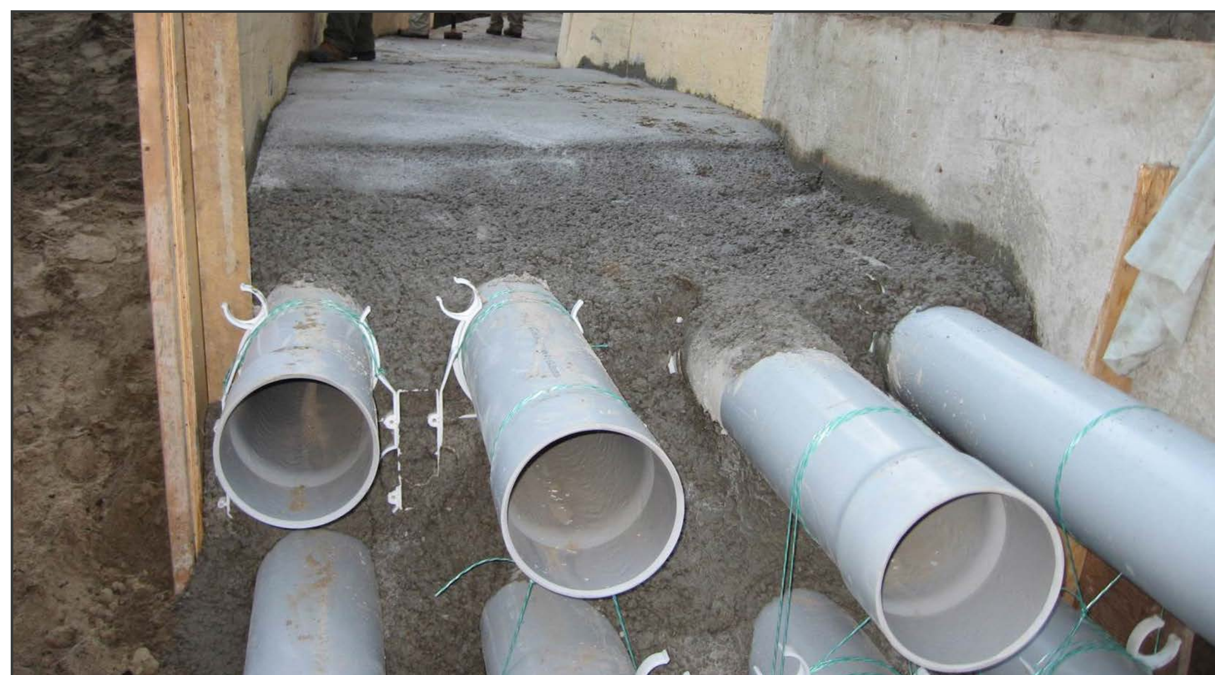
Example of cable ducts
