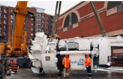
Photo of tunnel boring machine at Esplanade TS before it was lowered underground in January 2023.
