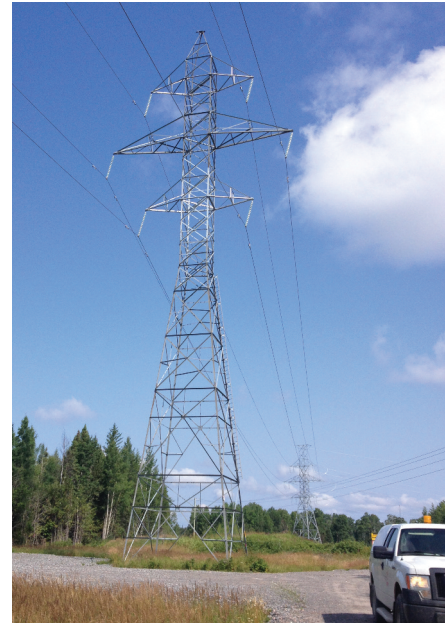
230 kV line with double circuit
