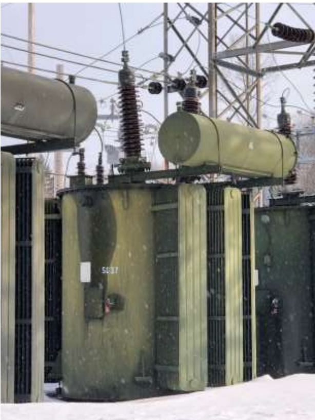
Goulais T1 with signs of oil leak
