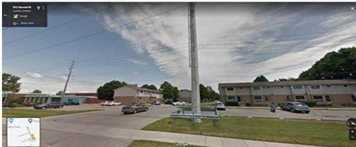
Figure 5 - Steel Tower carrying 230kV double circuits with guardrails around it
