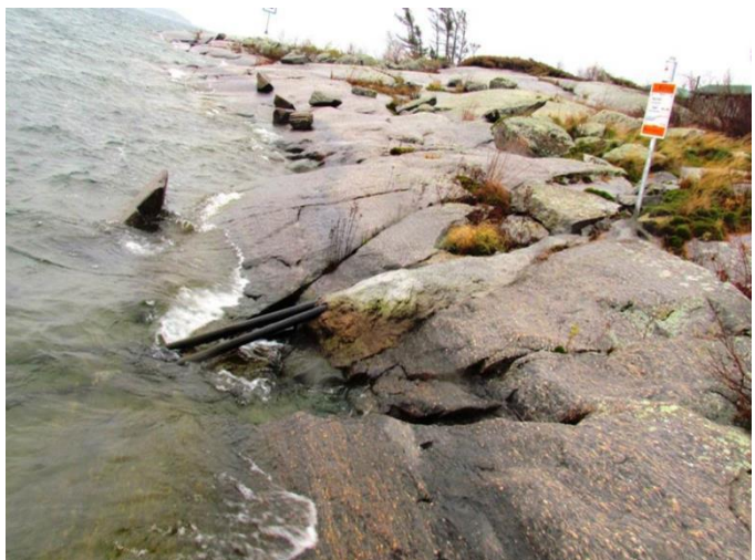
Figure 35 – Picture of Submarine Cable Entering Entering Water
