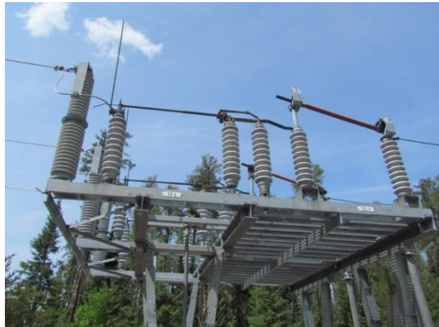
21 Figure 22 – Picture of Station Switch and Fuse Combination
