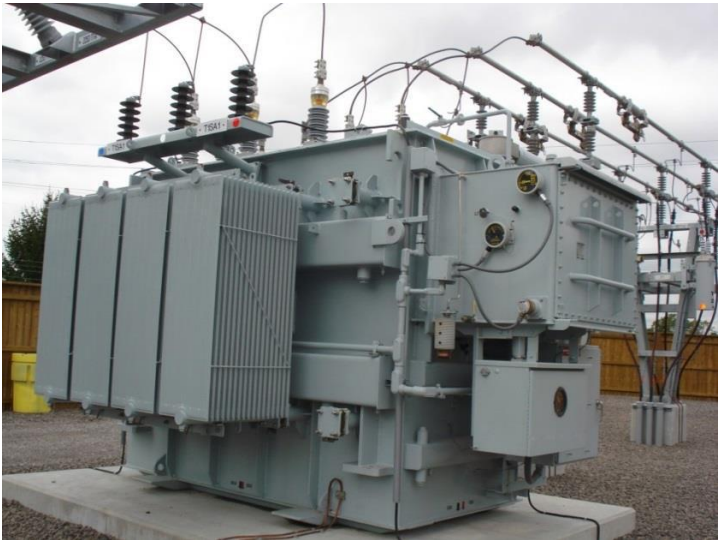
11 12 Figure 15 – Picture of Station Transformer
