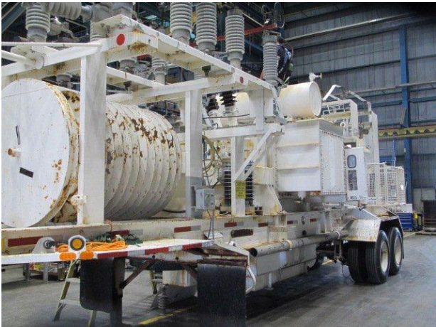
Figure 23 – Picture of Mobile Unit Substation
