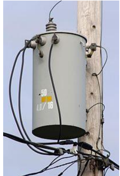
Figure 33 – Picture of Pole-Top Line Transformer
