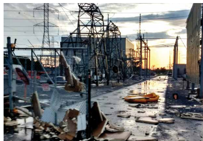
Merivale Transmission Station near Ottawa after a tornado destroyed the facility on September 21, 2018.
