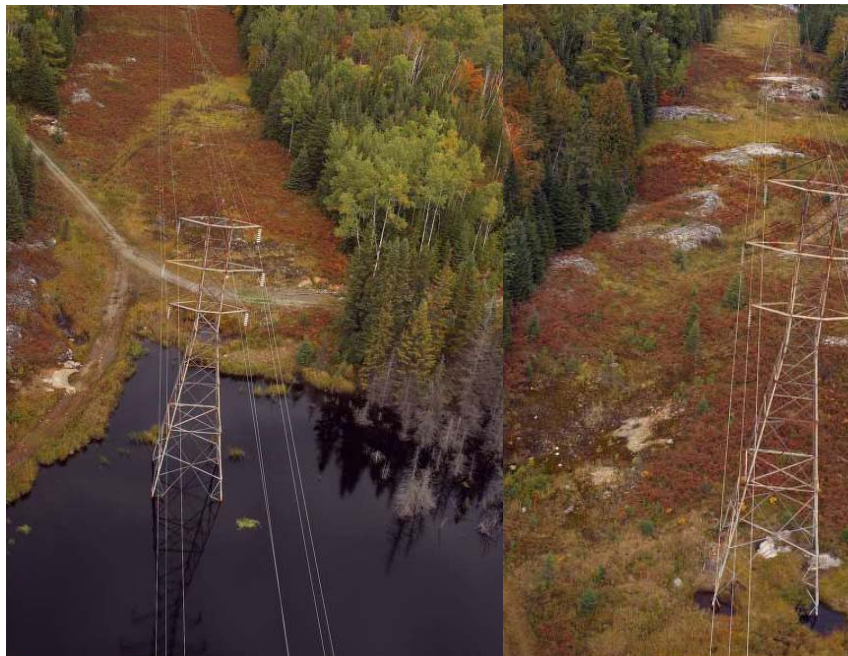
14 15 Figure 1 - Towers sitting in water causes the foundations to corrode, leading to 16 towers leaning (circuit D2L, near North Bay, ON)
