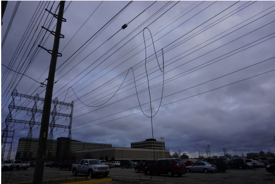
Figure 4 - V76R Insulator Failure
