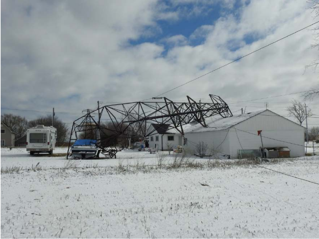
1 Figure 4 – 2018 K2Z (Haycroft DS x Belle River Jct) Steel structure failure
