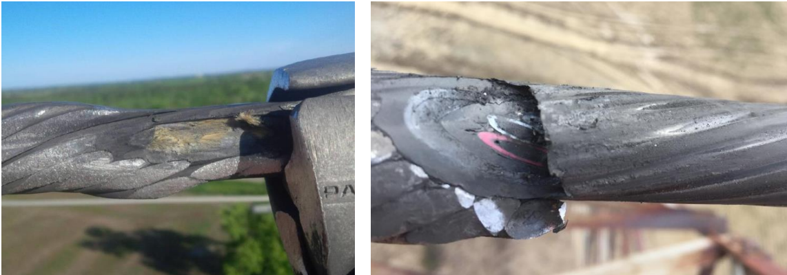
Figure 1 – ADSS Fibre Optic Cable Damage in 2017
