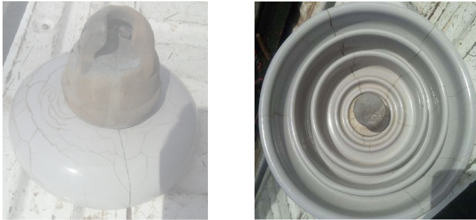
Figure 33 - Porcelain Insulator Unit Affected by Cement Expansion
