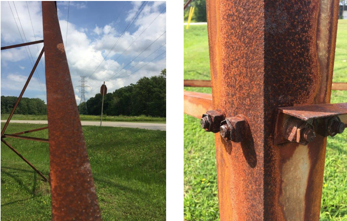
1 Figure 1 - Steel Structures in the Sarnia area exhibiting heavy pitting corrosion
