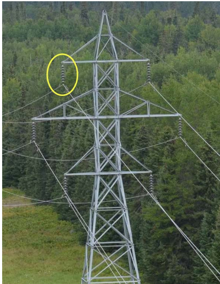
Figure 1 - Transmission Line Insulator
