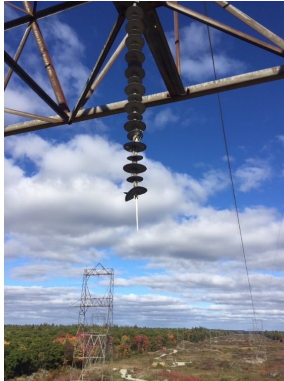
Figure 10 - Failed Polymer Insulator
