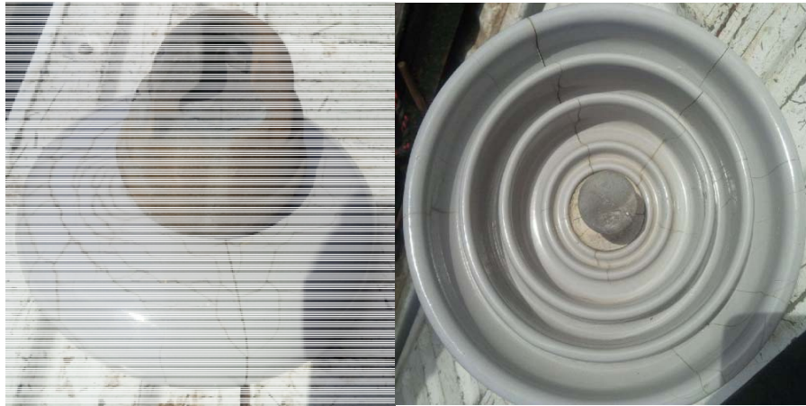
Figure 3 - Porcelain Insulator Unit Affected by Cement Expansion
