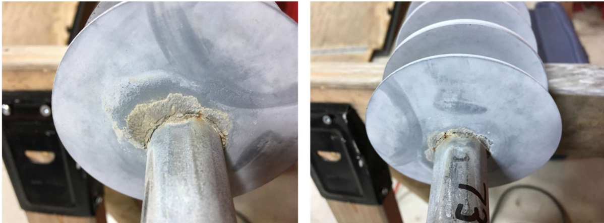
Figure 4-5 Damage to OB insulator line-end rubber and seal observed with no corona rings
