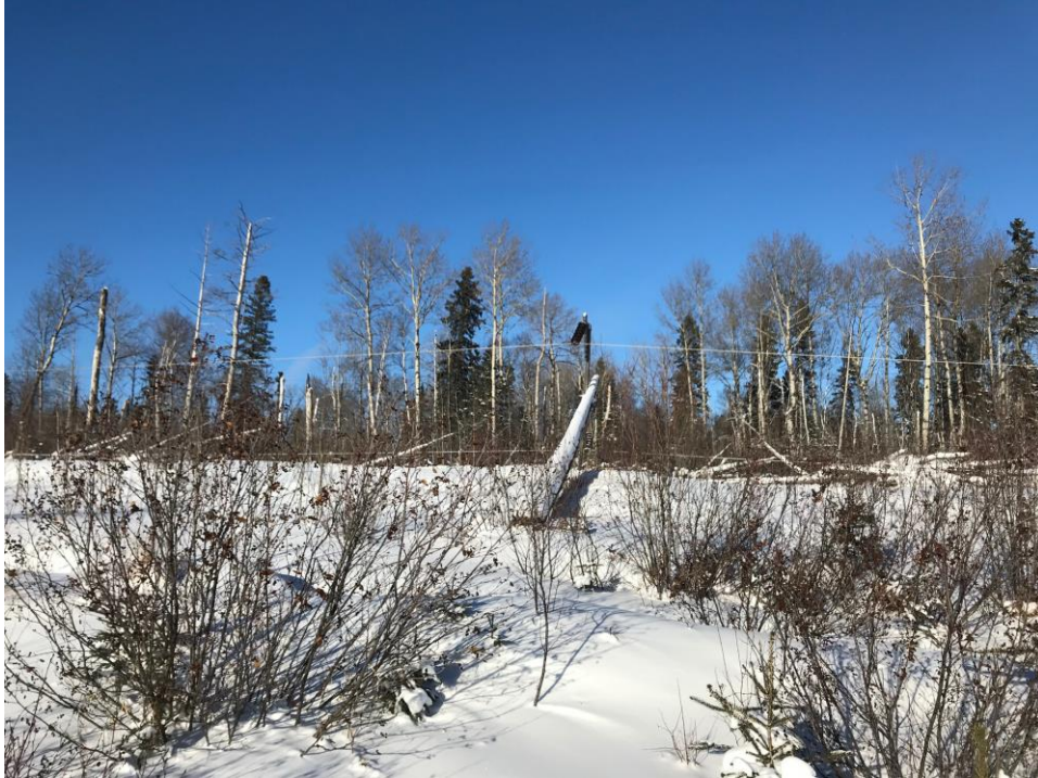
3 Figure 2 - Downed wood pole on circuit M1T
