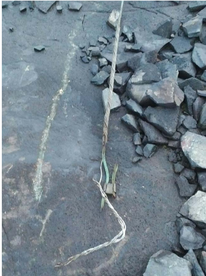
1 2 Figure 5: 2017 Shieldwire Failure on S22A 3
