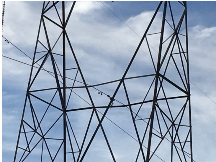
Figure 9 - Failed Polymer Insulator
