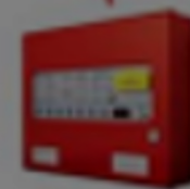
Fire Alarm Control panel
